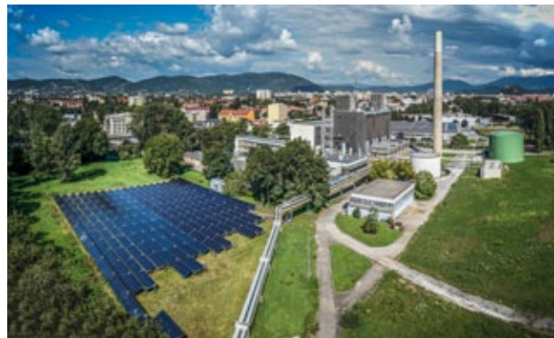
2014 installed field of solar collectors (2480 m 2 ) at the area of AEVG-Fernheizwerk Graz, Photo: S.O.L.I.D.
